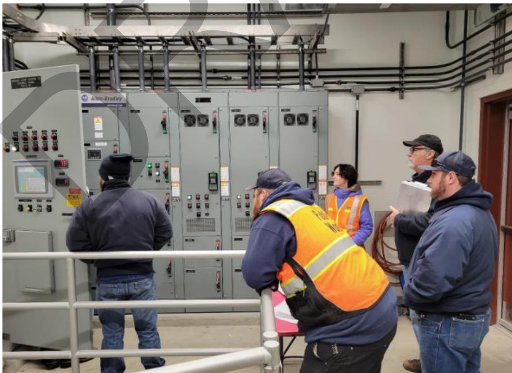
FIGURE 15: LIFT STATION 13 CONTROL ROOM
