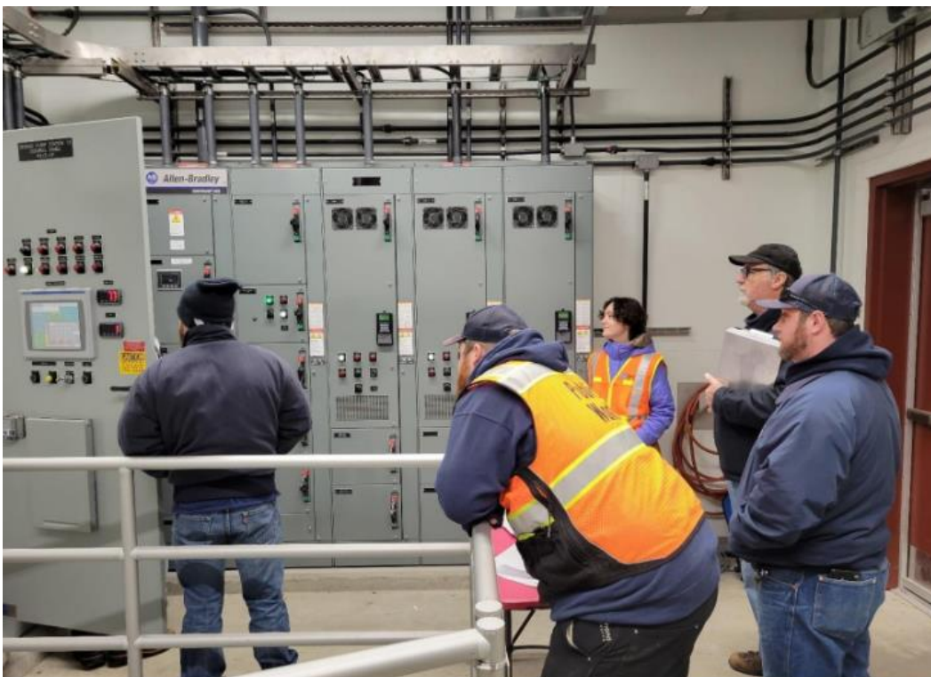
FIGURE 15: LIFT STATION 13 CONTROL ROOM
