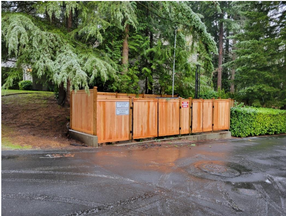
Wastewater Lift Station 15 after project completion
