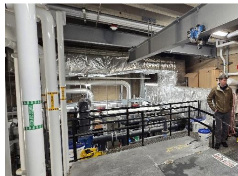
Mechanical, electrical, and plumbing equipment at the Redmond Pool
