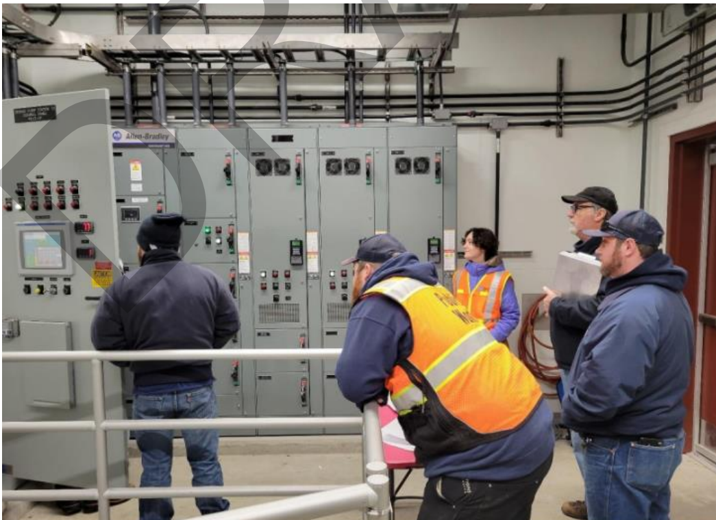
FIGURE 15: LIFT STATION 13 CONTROL ROOM
