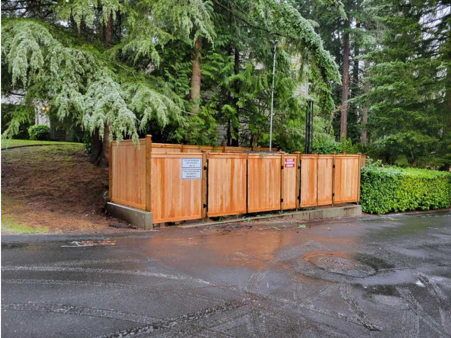
Wastewater Lift Station 15 after project completion
