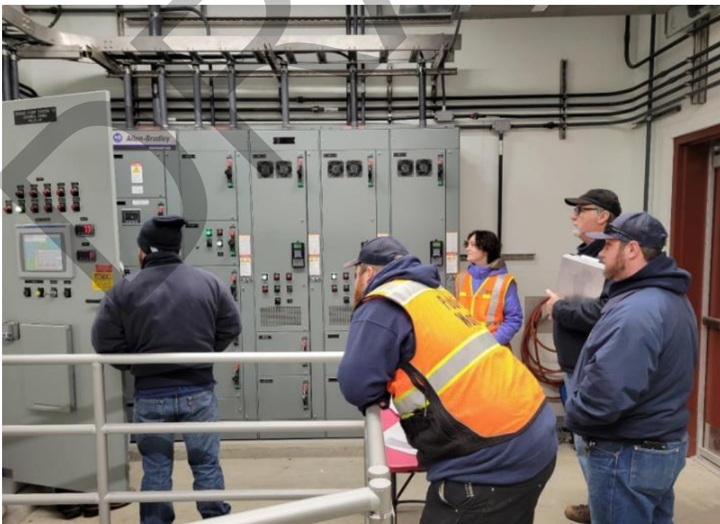
FIGURE 15: LIFT STATION 13 CONTROL ROOM
