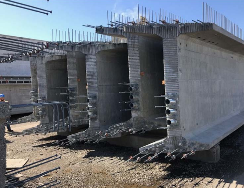
"I" girders ready to ship to the site 8.5' high, 4.3' wide, 161' long, 127 tons
