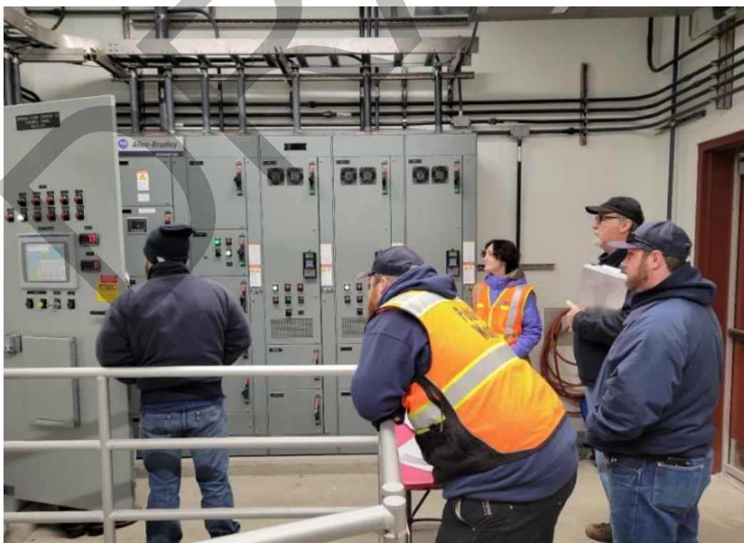
FIGURE 15: LIFT STATION 13 CONTROL ROOM
