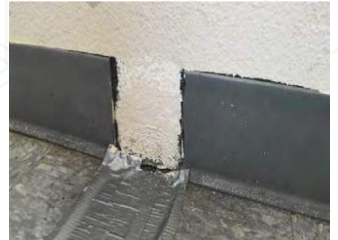
Asbestos Mastic Behind Rubber Base
