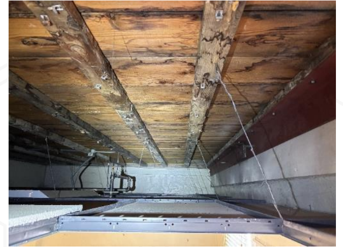
Water-Damaged Roof Deck
