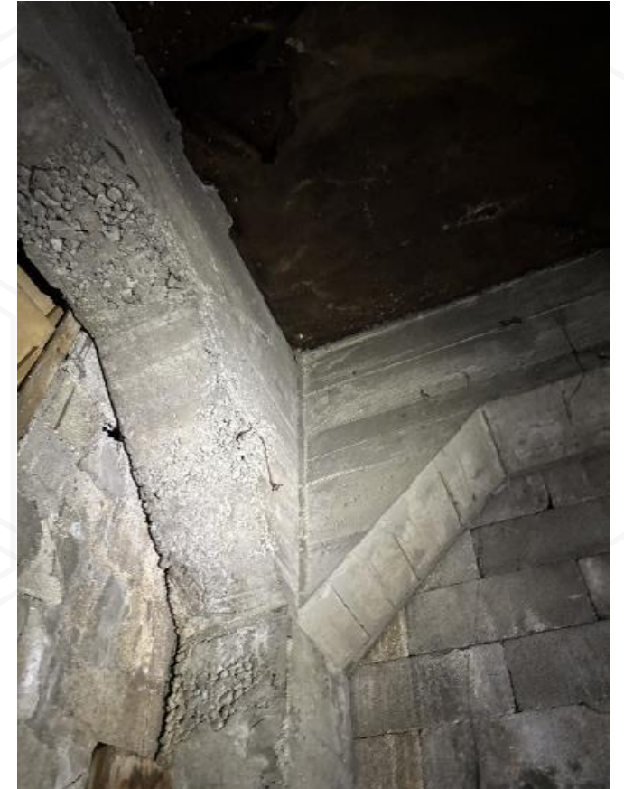
Hose Tower - Unreinforced CMU on Worn Concrete Frame
