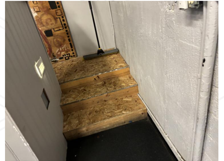
No Handrails and Non-Uniform Risers
