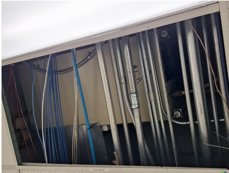
Figure 2 – WSHP 5A (located in ceiling plenum)
