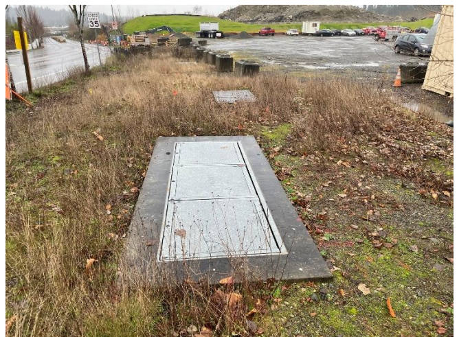
Photograph 12. Utility vault located west of the Property.
