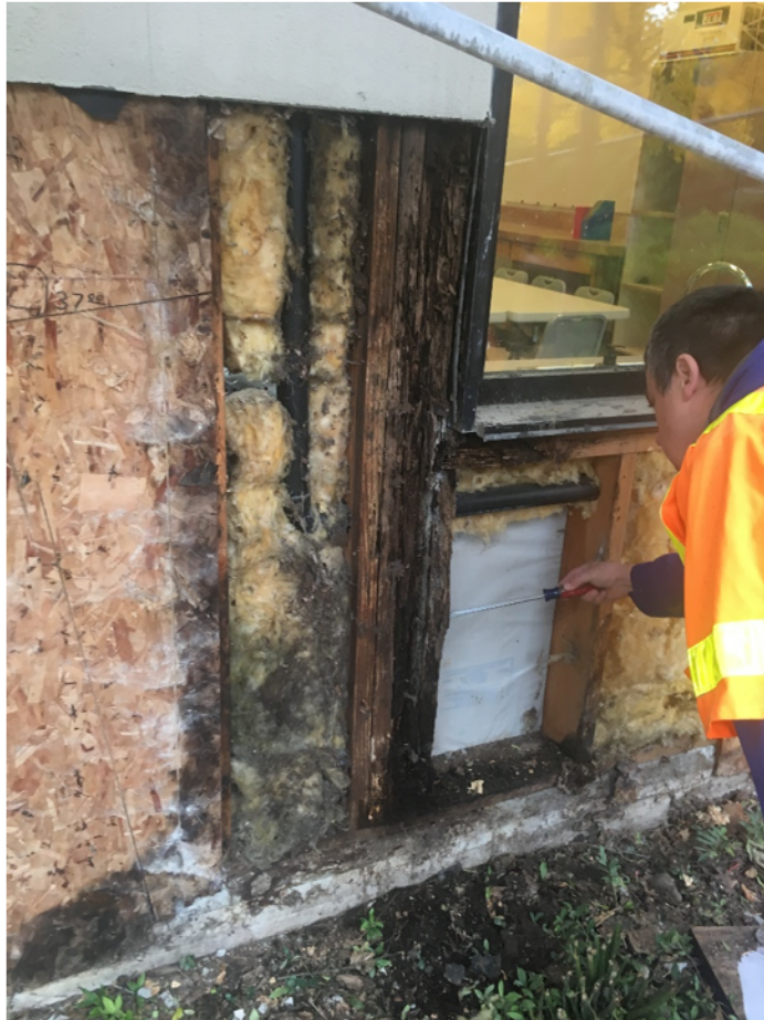
Figure 8. Moisture/dry rot damage at window sill plate without a sill pan flashing
