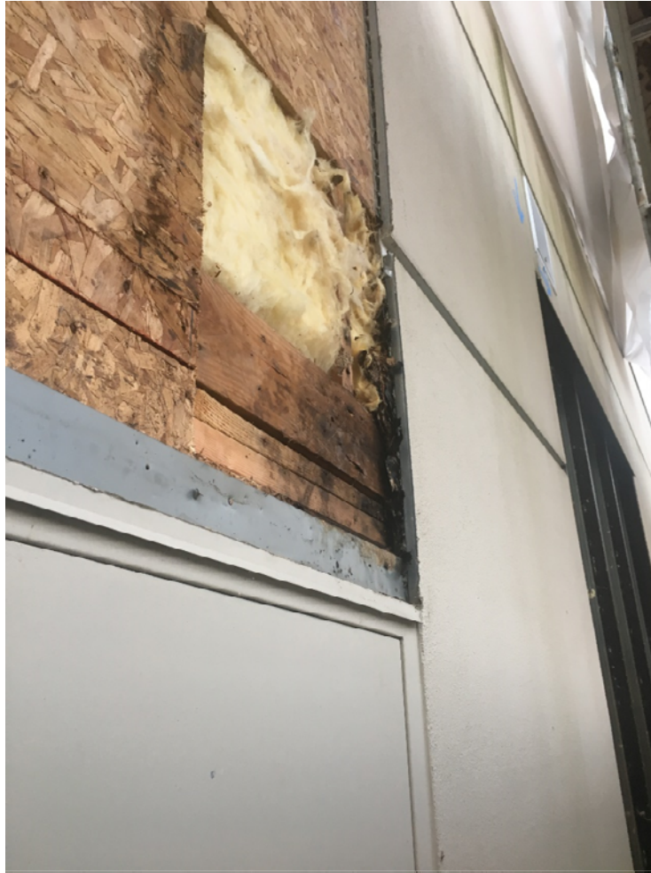
Figure 9. Moisture/dry rot damage behind trim joint above door head flashing
