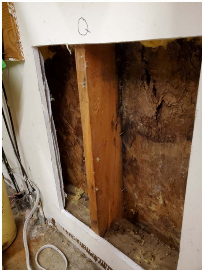
Figure 1. Damage at south wall
