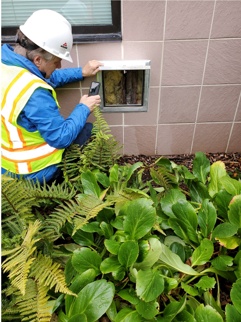
Damage at base of shearwall sheathing
