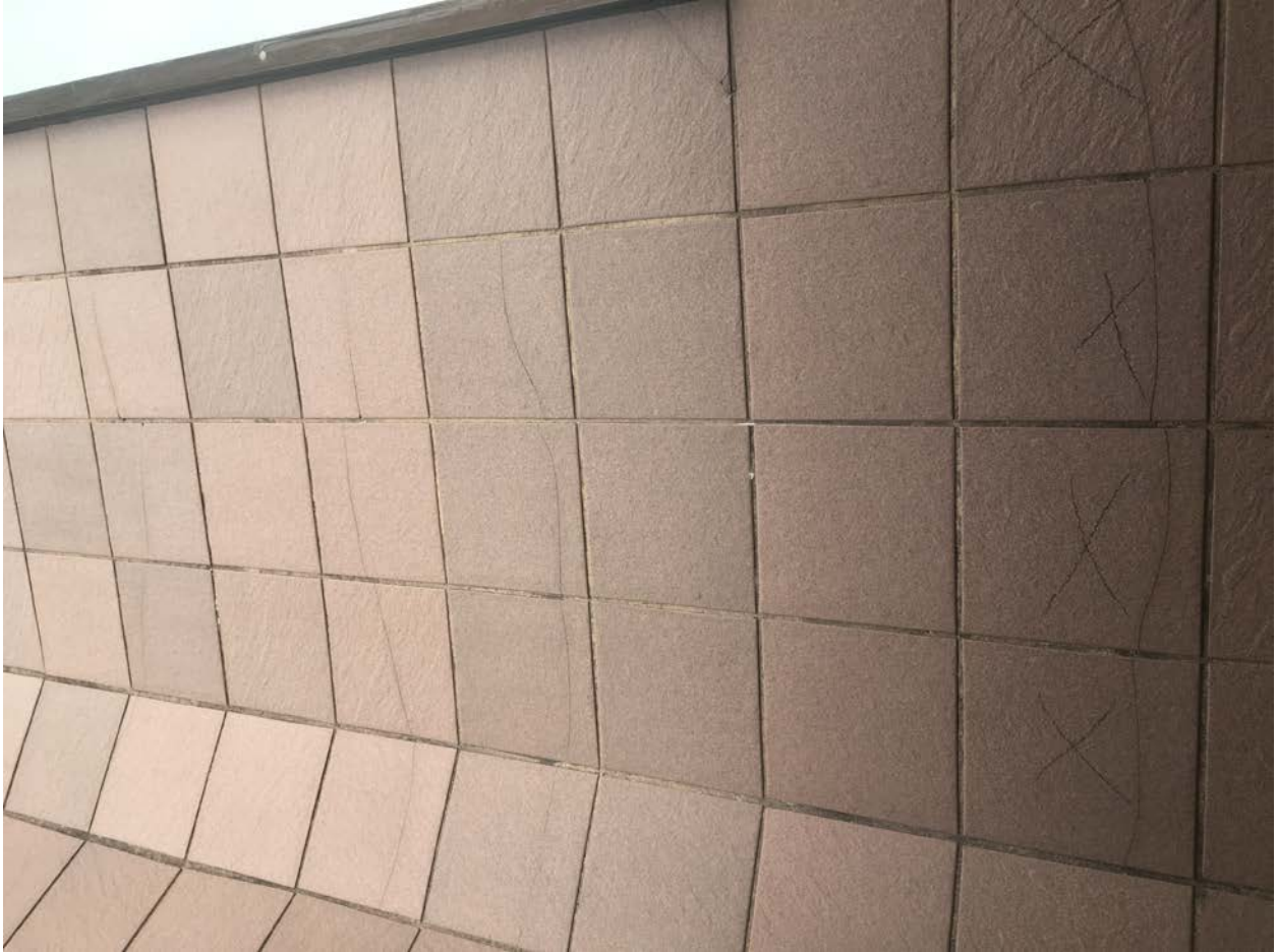
Tile cladding showing cracks. Moisture has gotten behind the tile causing cracks from thermal contraction and expansion.
