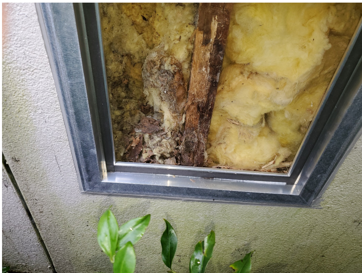
Damage at window jamb
