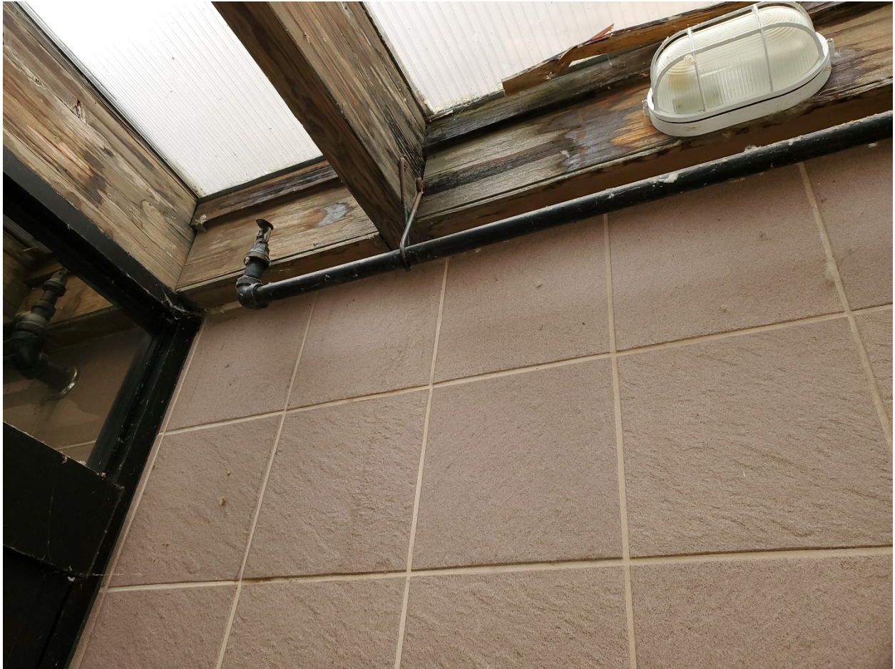
Closeup of front canopy framing damage
