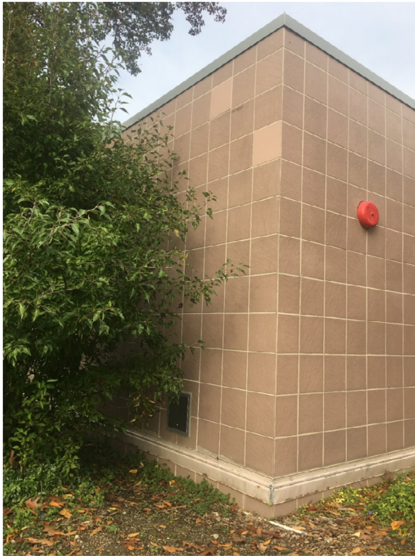
Figure 10. Tile cladding termination at soil in planter
