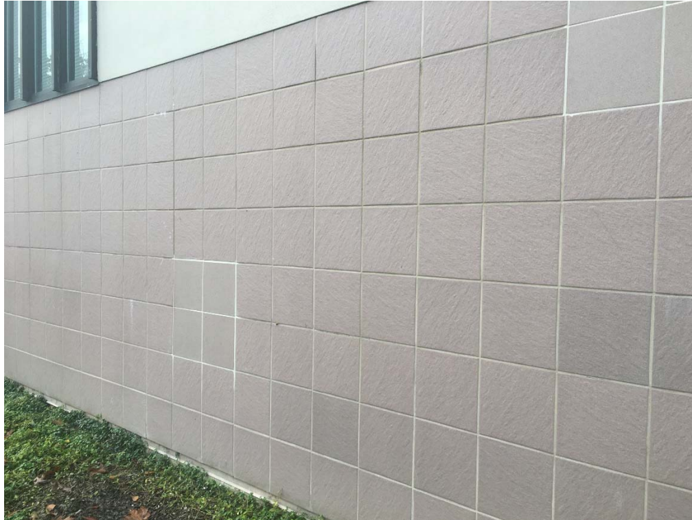
Figure 13. Lack of transition flashing at tile and stucco cladding intersection
