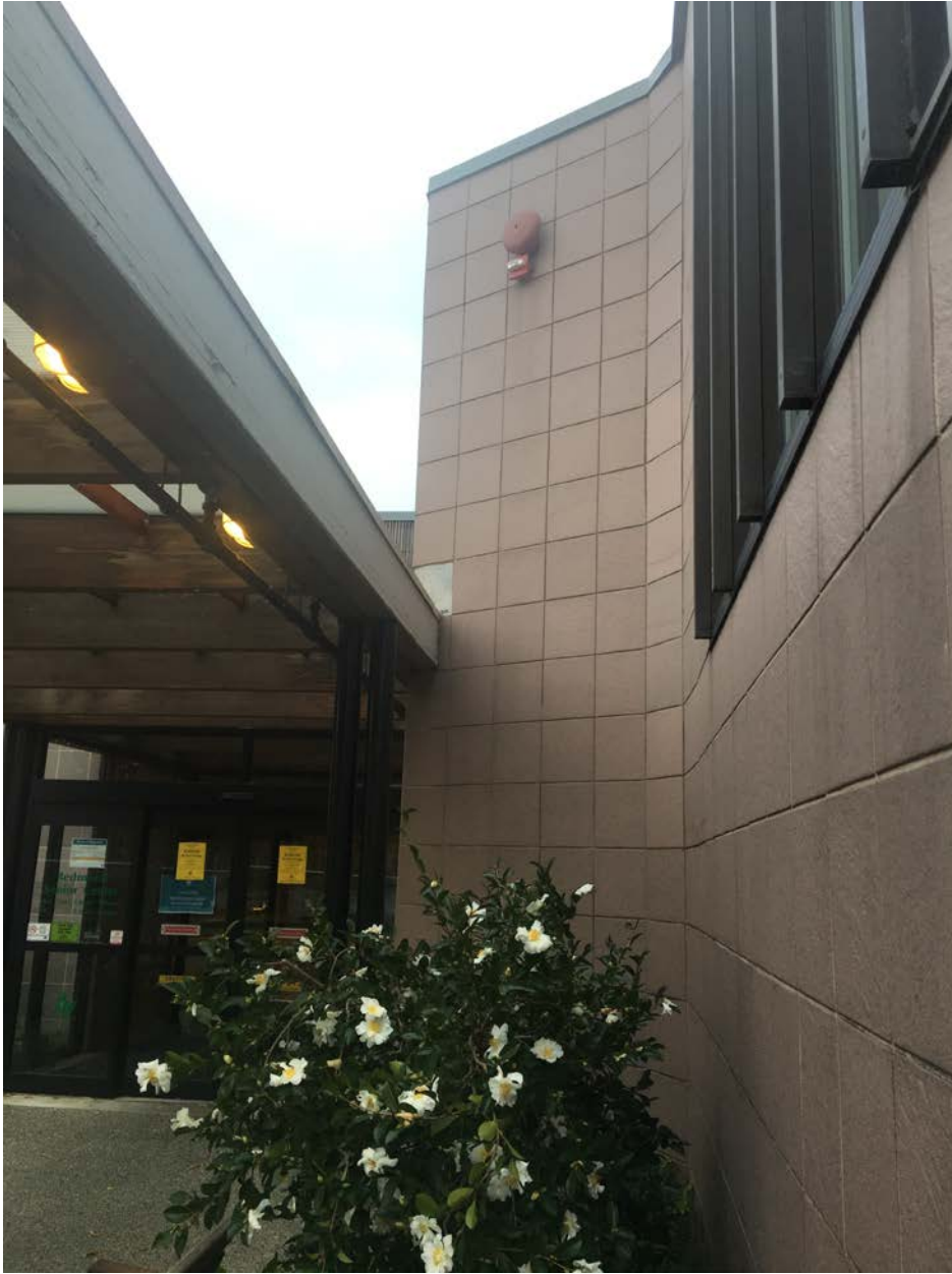
Tile above entry canopy has fallen off exposing mortar bed.
