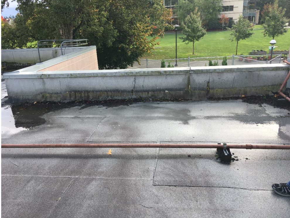
Figure 14. Roof showing evidence of slow draining and ponding
