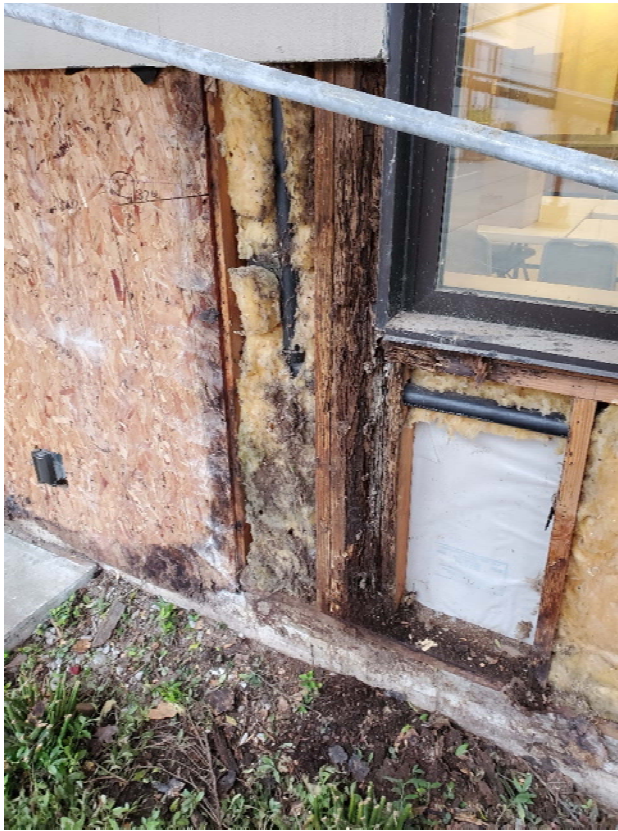
Figure 3. Damage to framing, base plates, and windowsill
