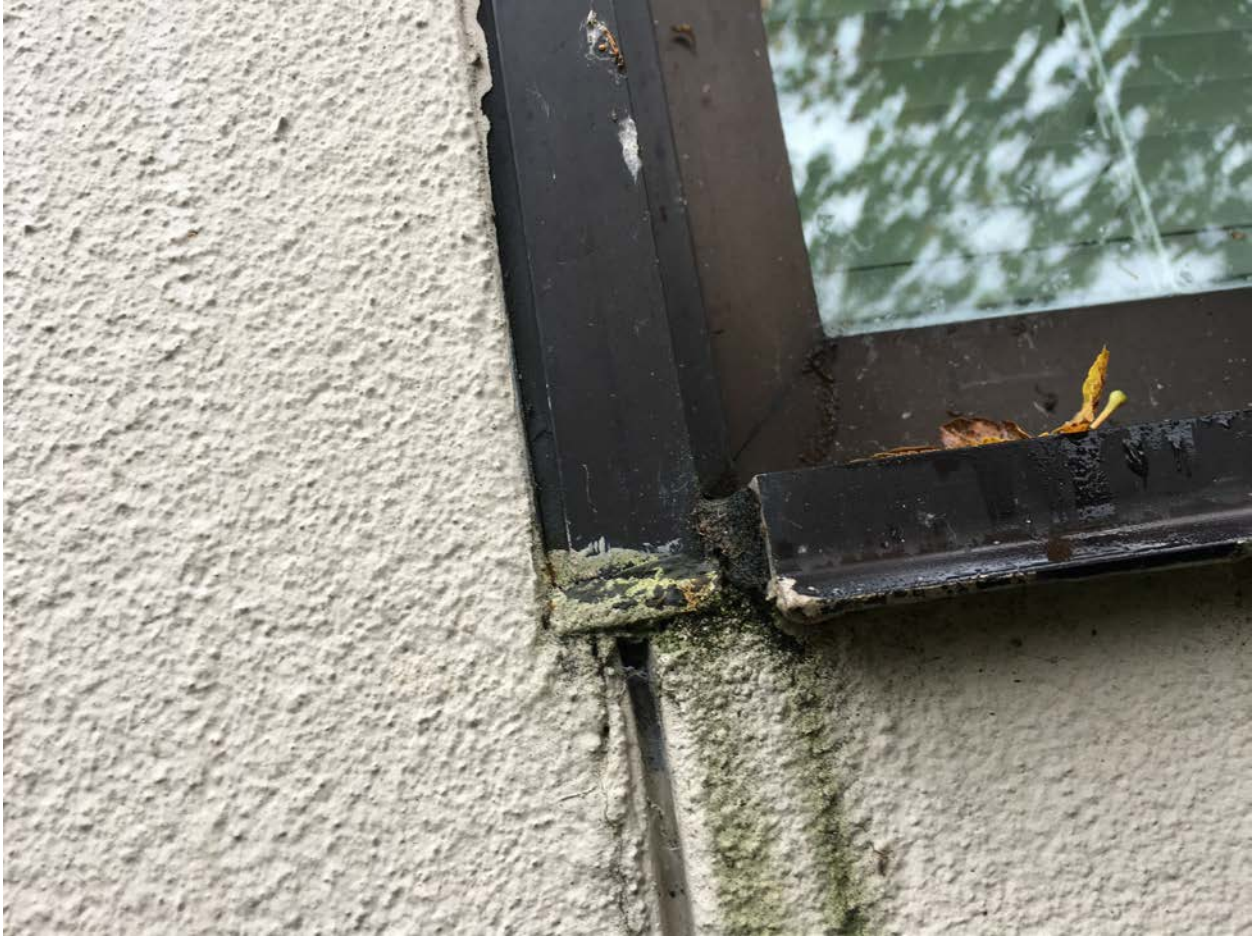
Sill flashing without sill pan and sill end dams. Sealant at corner is the only protection from moisture/dry rot
