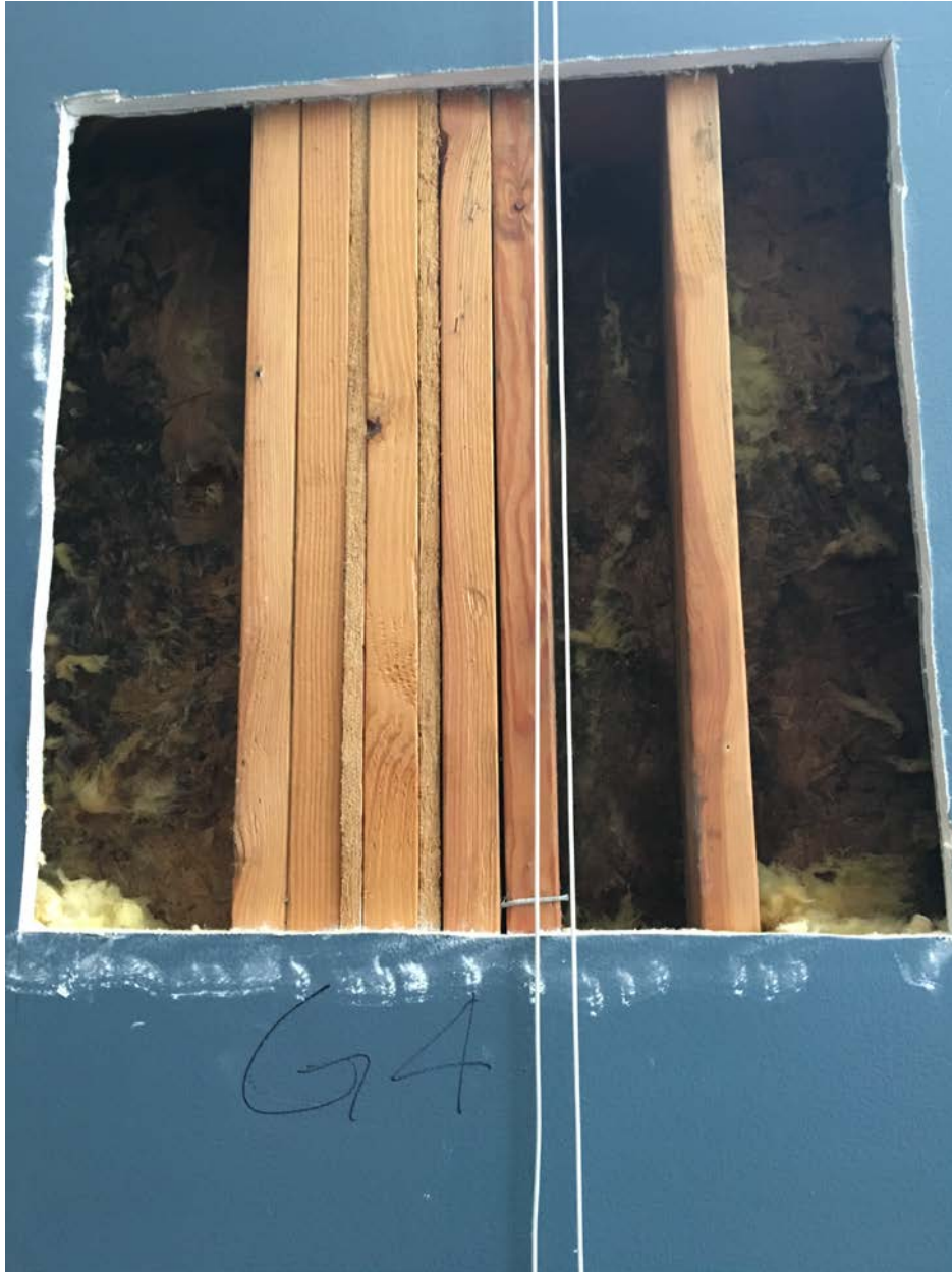
Access port cut in east wall of Meeting Room (208) showing moisture / dry rot at stucco cladding intersection.
