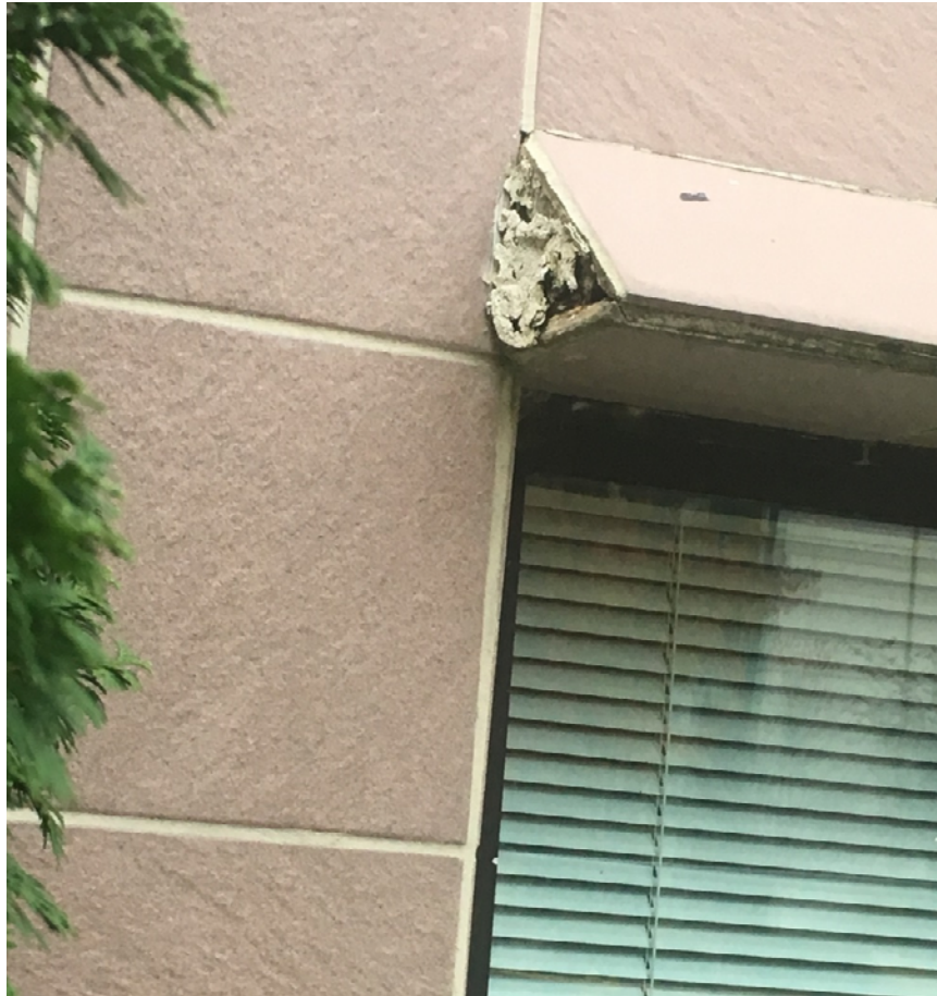
Figure 11. Tile cladding showing damage at window head
