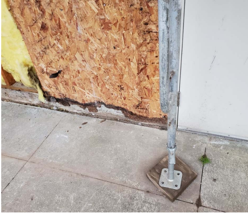
Figure 2. Damage at base of shear wall sheathing
