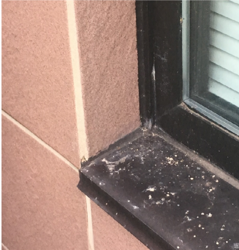
Figure 12. Sill flashing without end dam and sill pan
