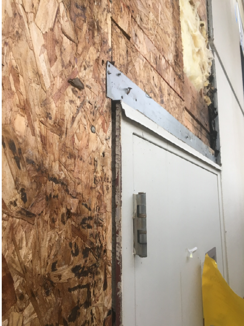
Figure 7. Lack of end dam at head flashing above door frame
