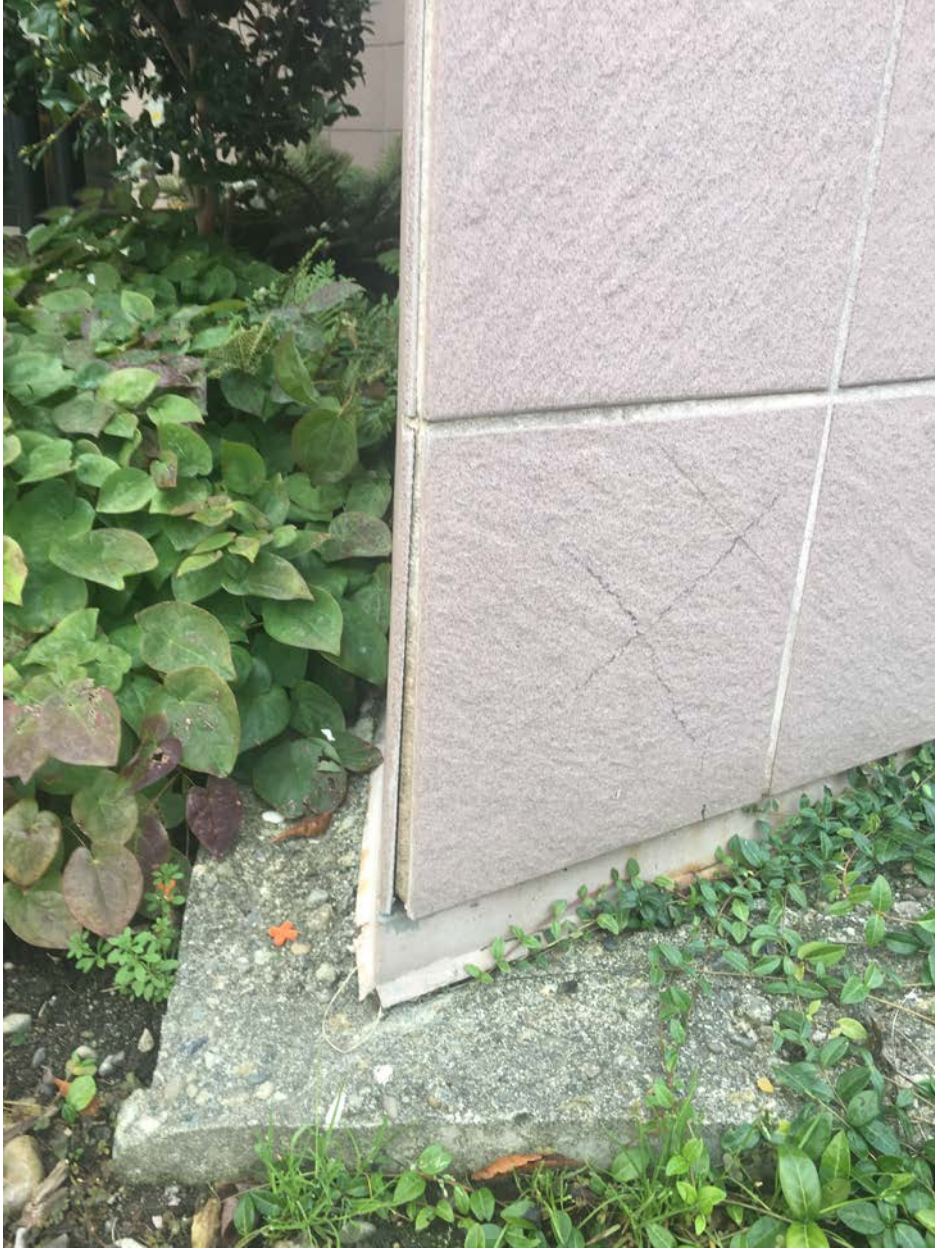
Tile cladding marked for replacement. Tile has pulled away from mortar bed.
