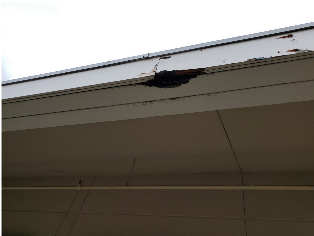
Damage at eave gutter to west of ballroom
