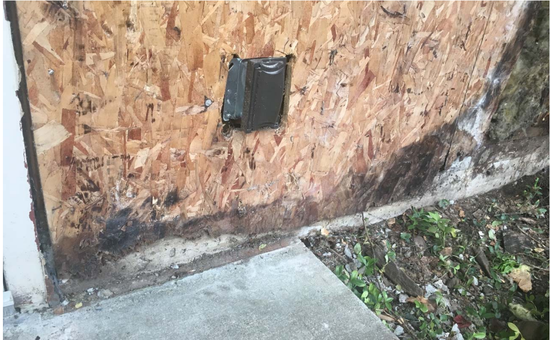
Figure 6. Moisture/dry rot at stucco cladding termination at sidewalk and soil.
