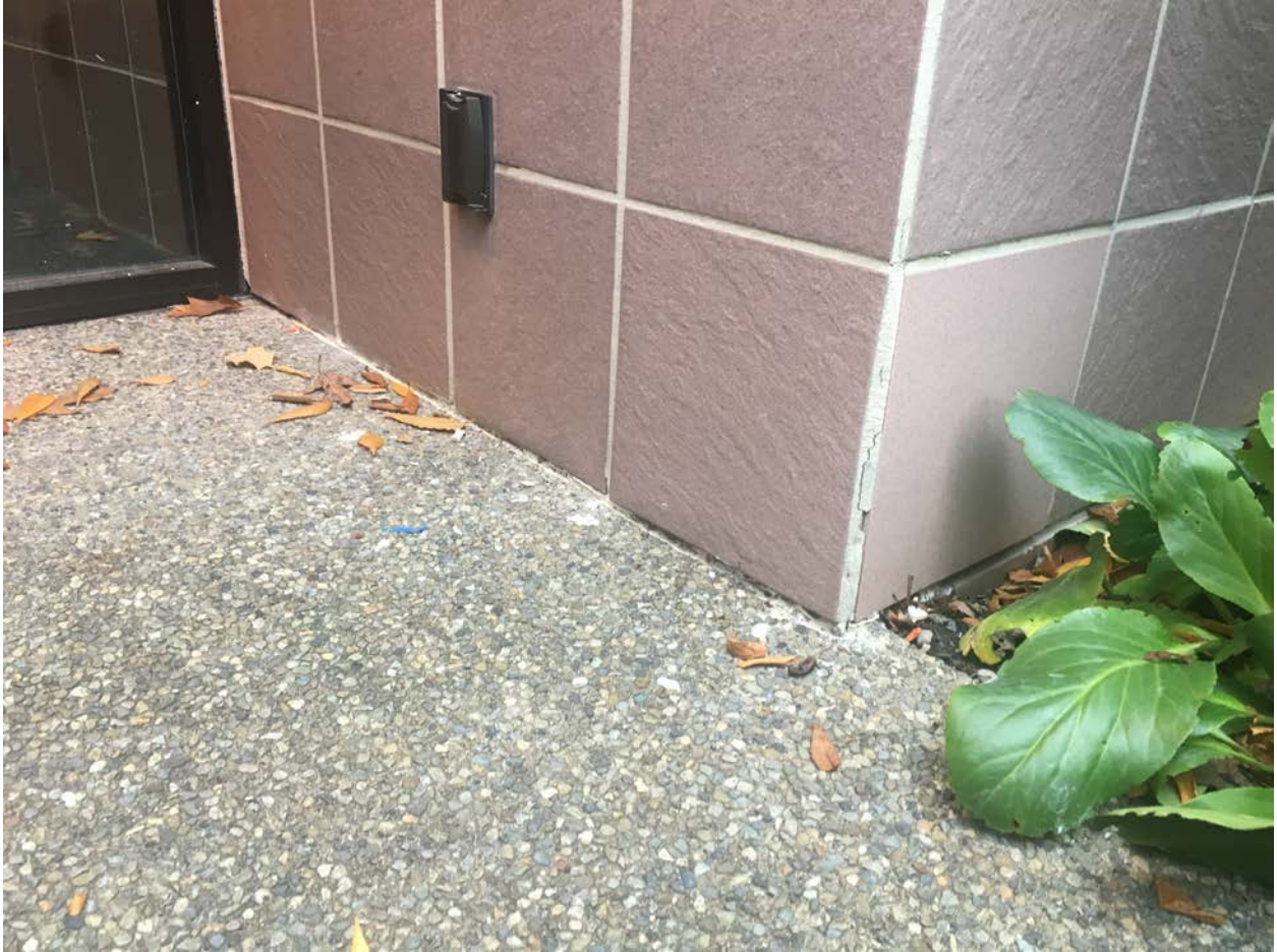
Tile at sidewalk without a 2" minimum gap and flashing. Tile grout at corner has failed and will allow moisture / dry rot to damage substrate.
