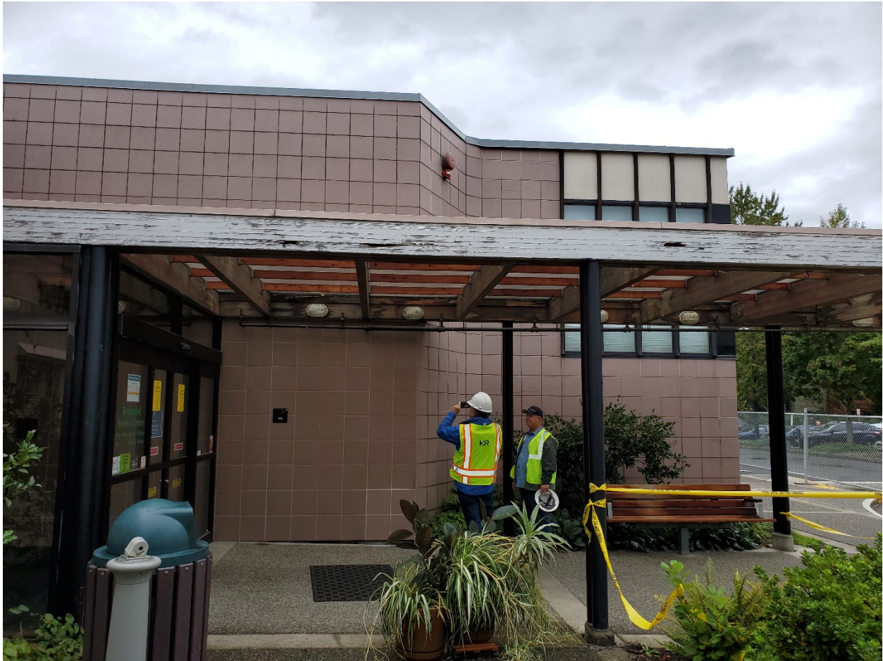
Damage at front canopy framing
