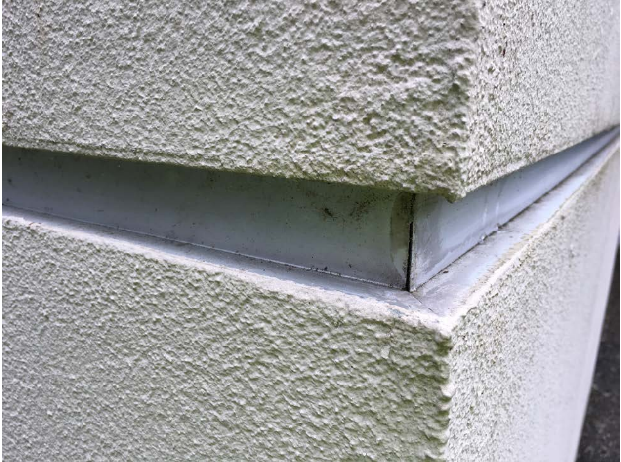
Stucco trim joint without factory molded outside corner. Moisture can enter at open corner joint.
