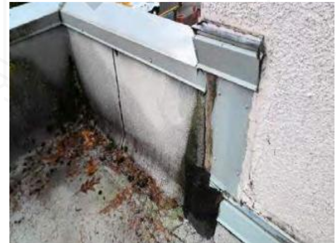
Water Intrusion at Failing Flashing
