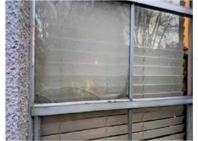
Original Windows Contain Lead Paint and Asbestos
